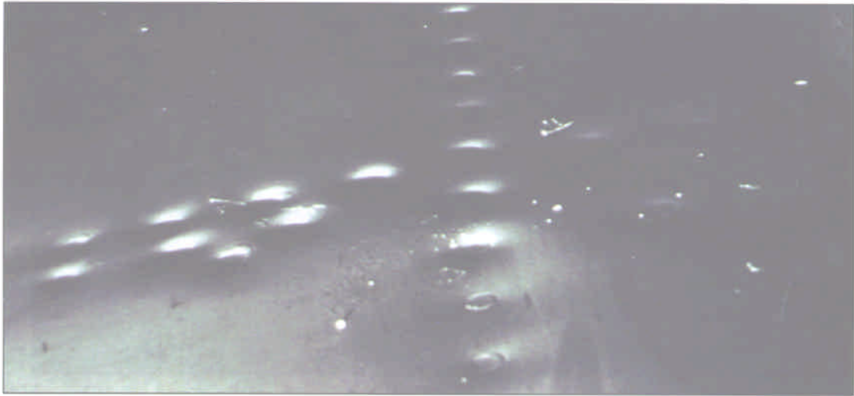
FIGURE 4-12. SKIN BULGING AROUND FASTENERS
